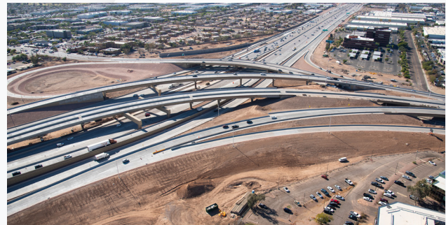
The SR 143 and I-10 interchange in 2024 after the new eastbound I-10 loop ramp to northbound SR 143 and the new southbound SR 143 ramp to eastbound I-10 opened.
