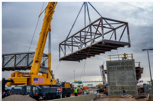
A crane lifts the piece of truss that will connect the multiuse bridge over I-10 to the west-side landing at Alameda Drive.
