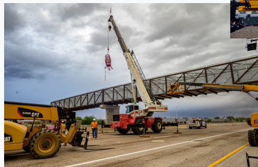
A crane lifts the prickly pear cactus fruit, so workers bolt it to the top of the bridge.
