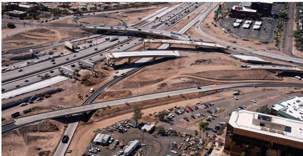
The SR 143 and I-10 interchange in 2023 when crews were constructing the flyover ramps.
