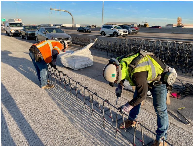
Workers tie rebar together for a barrier along eastbound I-10 near the Salt River.
