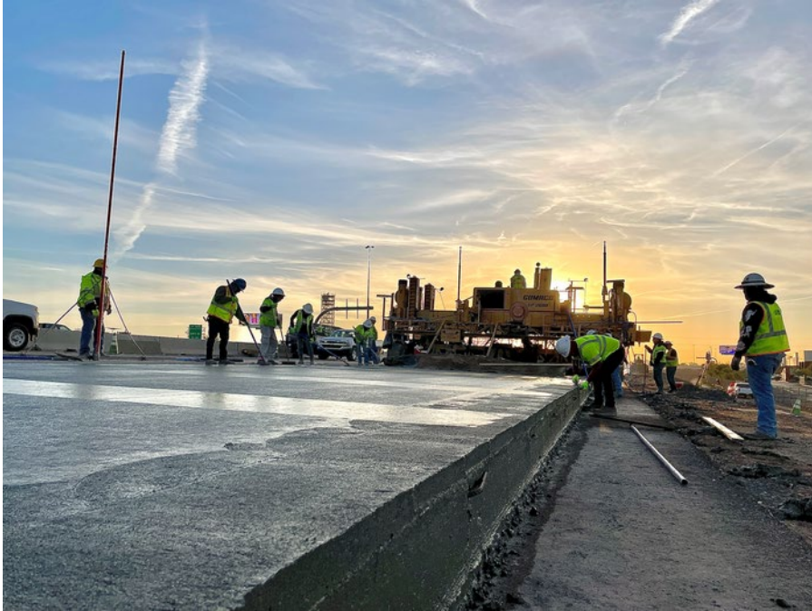
A paving crew places concrete to connect the new portions of the roadway into the eastbound I-10 bridge over the Salt River.
