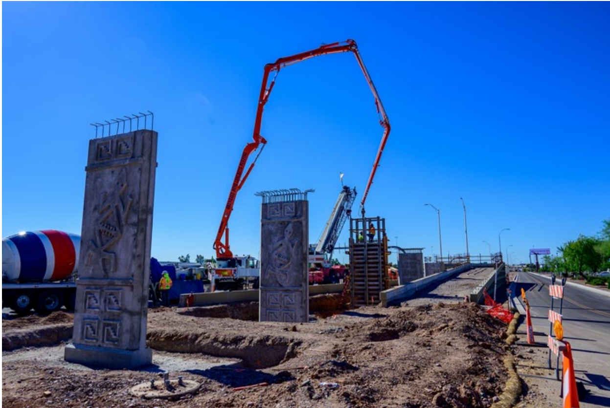
A concrete pump fills a support pylon for the west side of the multiuse bridge at Alameda Drive.
