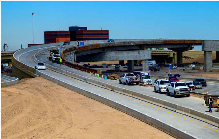
The ramp from southbound SR 143 to eastbound I-10 opened to traffic in late August, replacing the former loop ramp and improving the flow of traffic between the two roadways.
