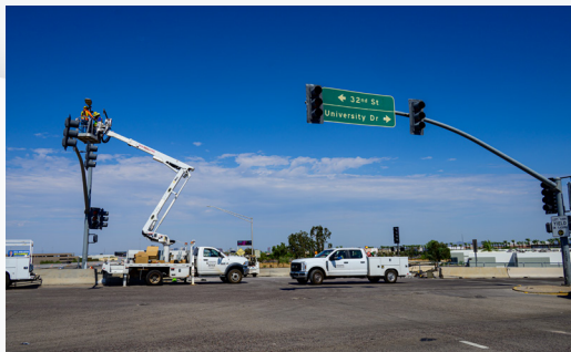
Crews work on overhead lighting and traffic signals in preparation to reopen the westbound I-10 on-ramp at 32nd Street.
