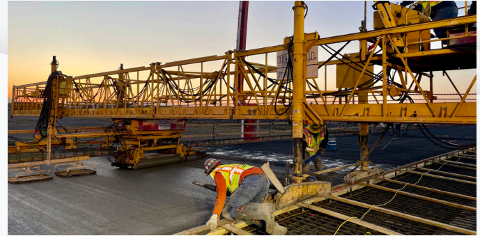
Workers place the concrete for the widening of the westbound lanes of I-10 over the Salt River.
