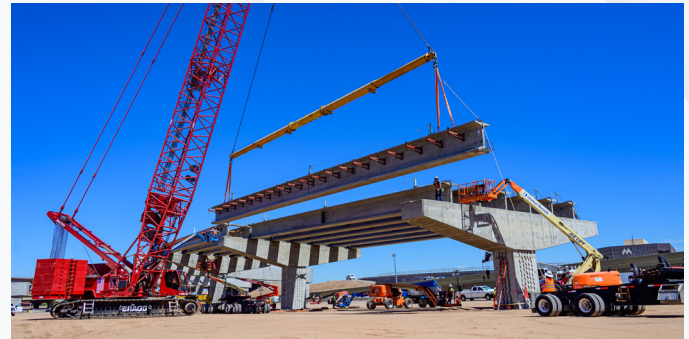
A crane sets a concrete girder for the high-occupancy vehicle (HOV) ramp that will connect I-10 with State Route 143.
