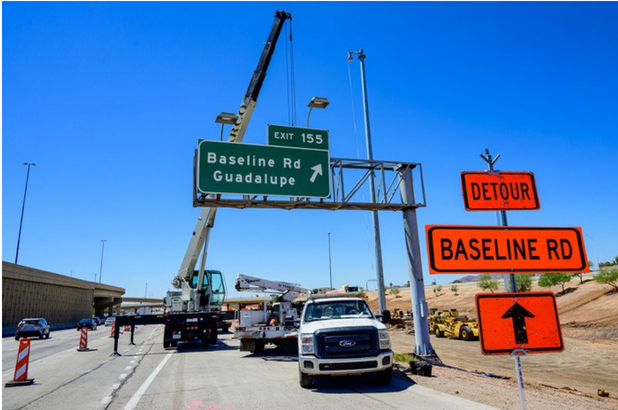
A crew removes the overhead sign following the closure of the eastbound I-10 off-ramp at Baseline Road.
