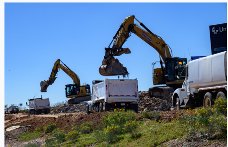
Excavators load the rubble from the eastbound I-10 off-ramp at 32nd Street into dump trucks to be hauled away.
