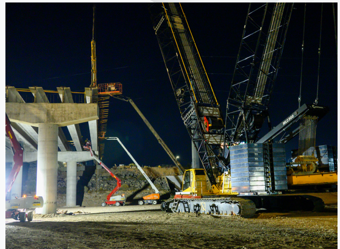
Once the girder is set, crews then make sure it is stable and secure before disconnecting it from the crane.
