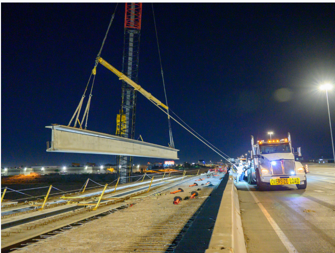
A crane lifts a girder from westbound I-10 and slowly moves it into position on the new bridge caps.
