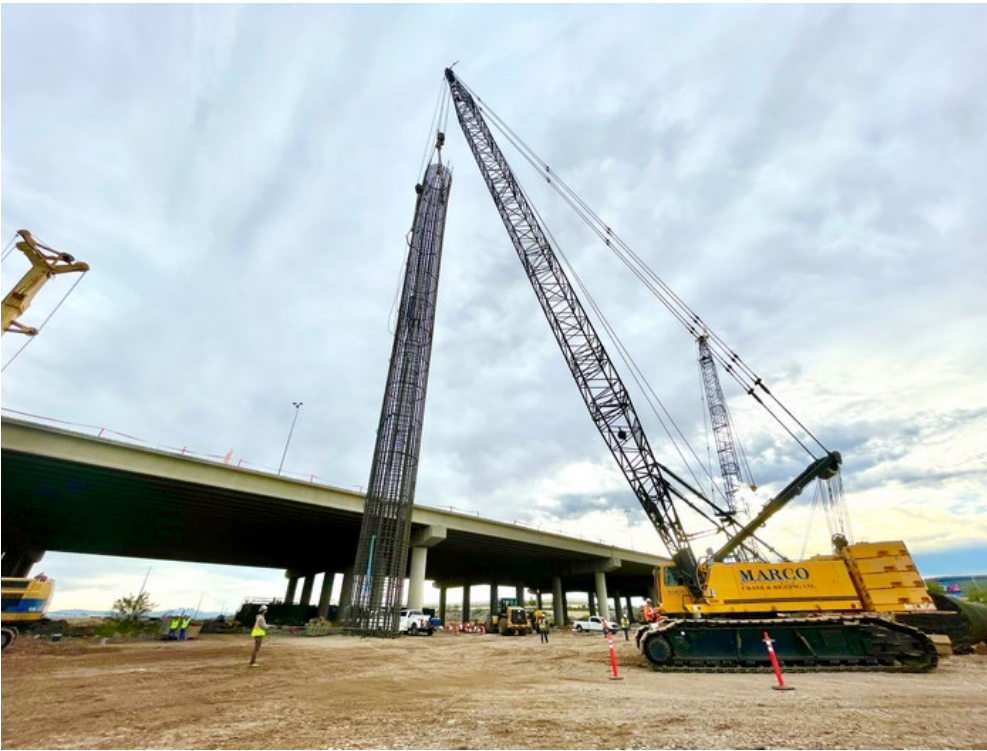
A crew uses a crane to install a drilled-shaft foundation rebar cage for the bridge that will widen eastbound Interstate 10 over the Salt River.
