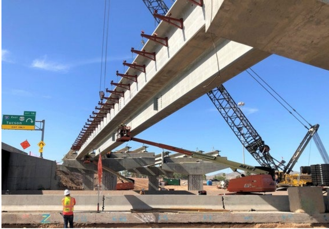
Above: Crews place girders for the new 48th Street bridges over I-10. See more pictures of girders being placed and other construction activity here .
